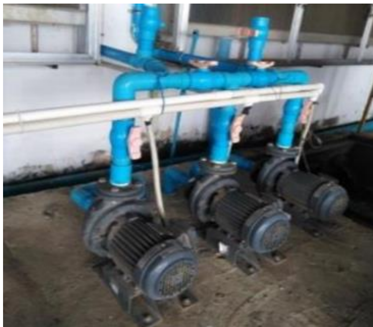
Water Pumps System
