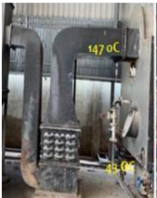
Uninsulated fuel gas duct
