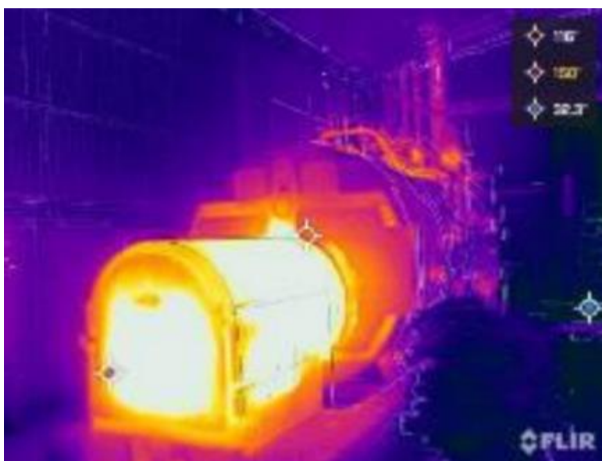
Temperature profile of boiler
