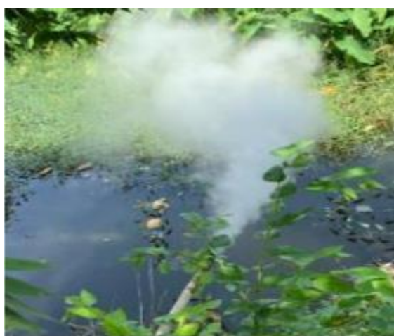
Condensate discharges out
