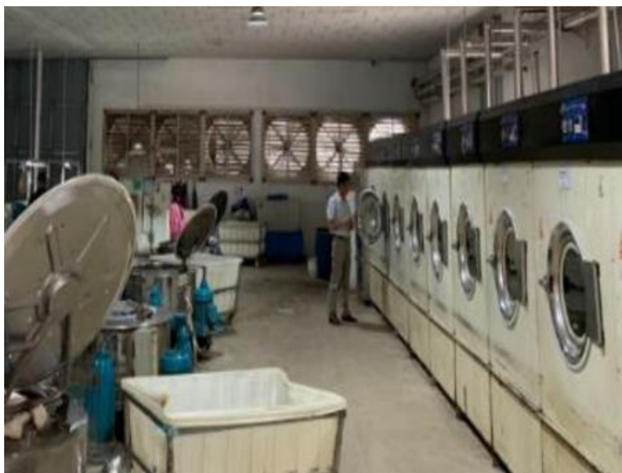
Air cooler fans in washing area
