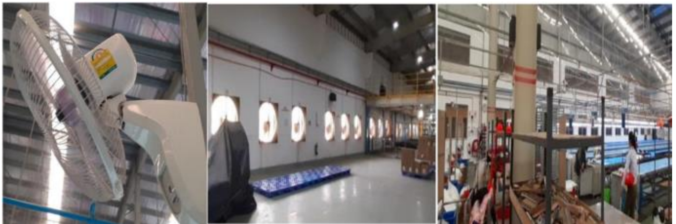
Space Conditioning System
