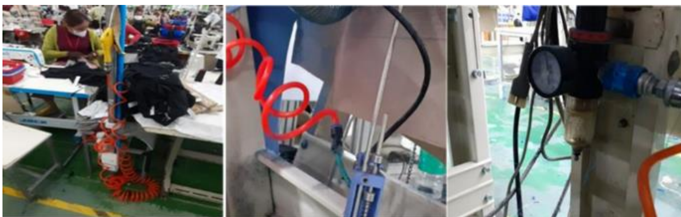
Compressed air tapping for sewing machines and cleaning lines
